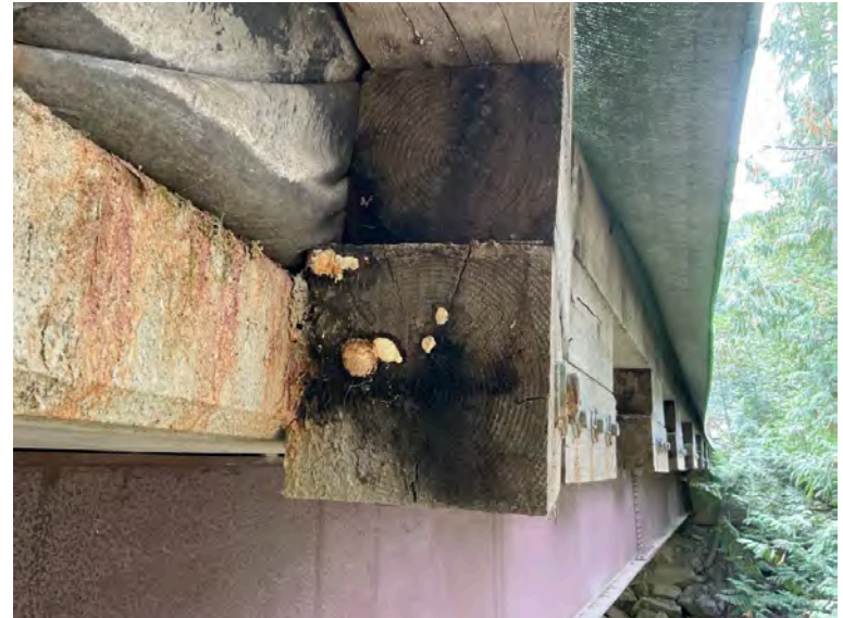
Guardrail sideblock condition
