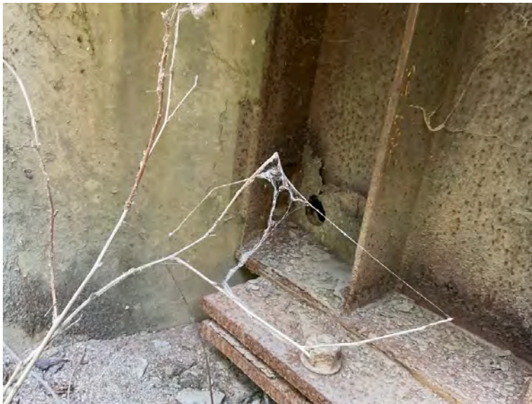
Upstream left bank steel corrosion
