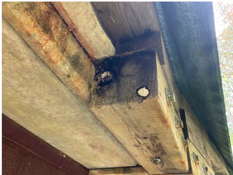
Guardrail sideblock condition
