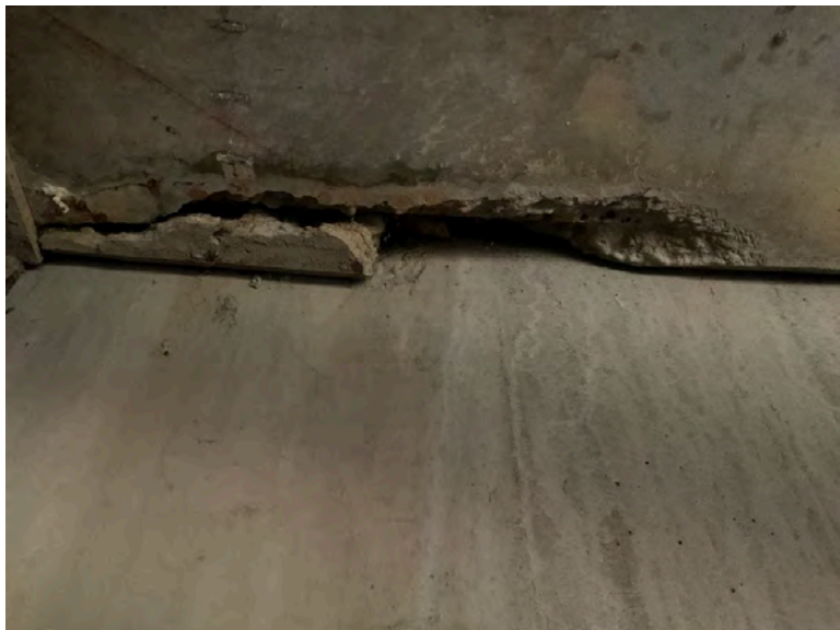
1st panel right bank damage
